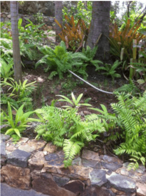
more pipes on owners road
