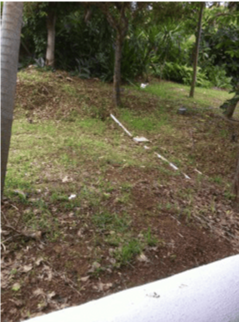
open pipes behind tiki
